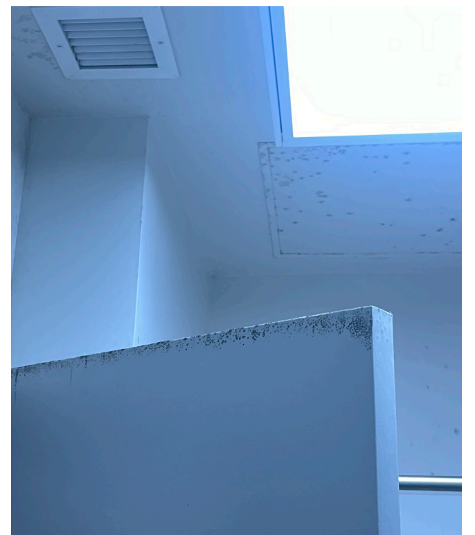
Mold in a dorm bathroom photo by Kaydence Hill
