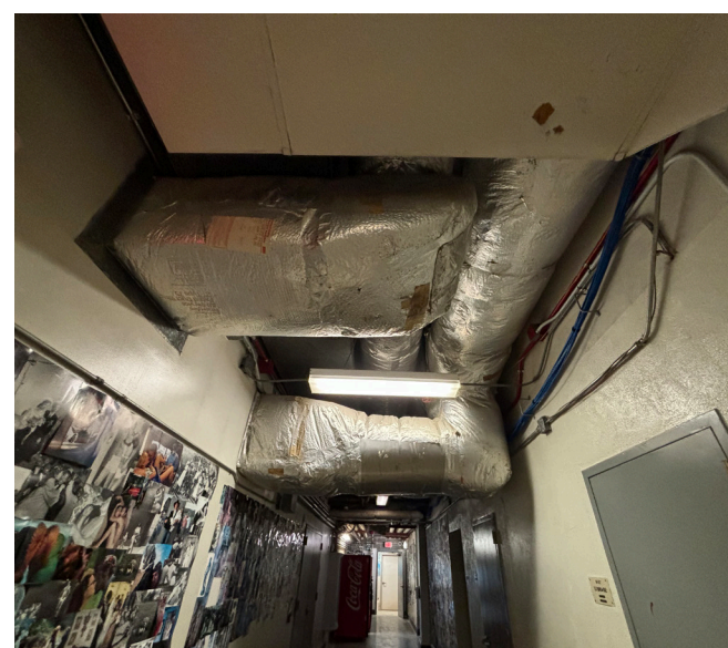
Photo of Rutledge's HVAC system photo by Clark Vilardebo
