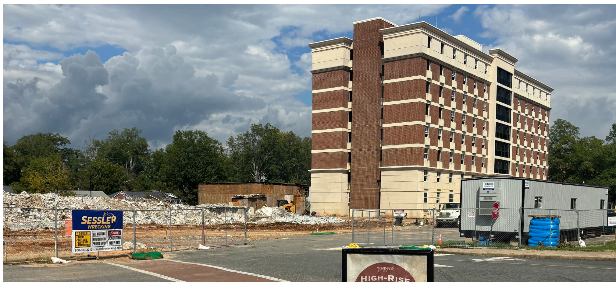
The remnants of Wofford Hall, with Richardson in the background
