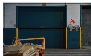
While it's being used as an elevator during construction, this area will eventually turn into the main stairwell connecting the lobby to the offices.
