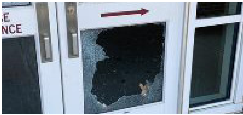
Deer broke through West Center glass door
